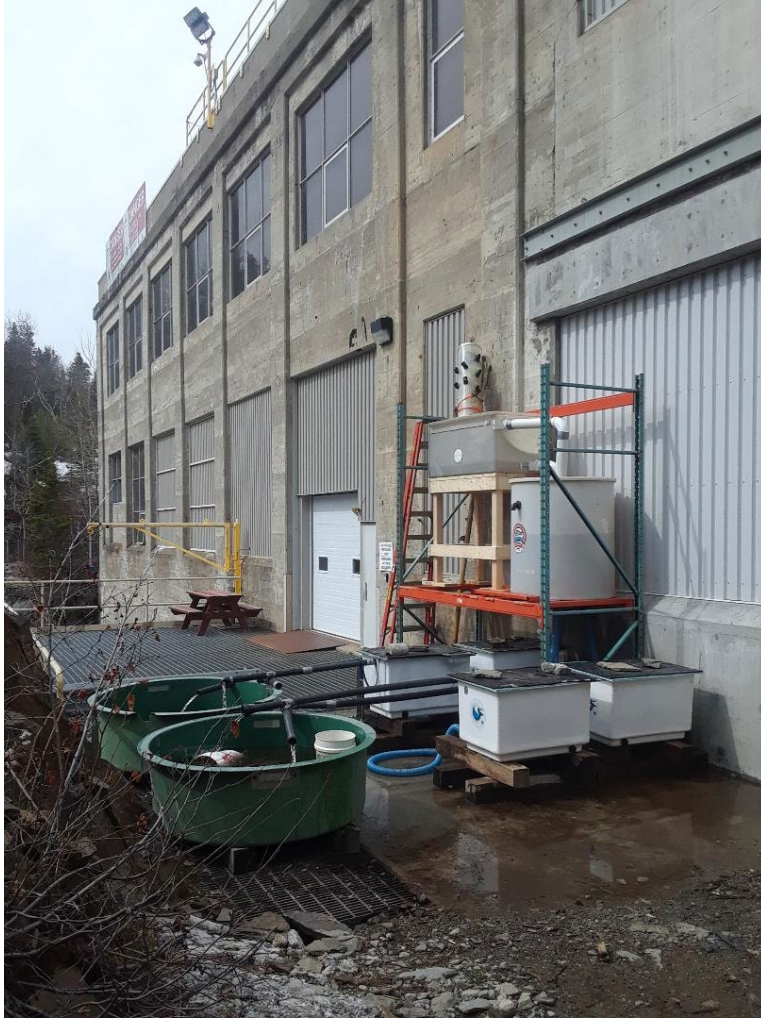
Photo 1: Stream side incubation system set up at the power dam
