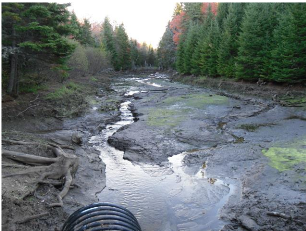
Before photo displaying effects of severe flow obstruction (2010)
