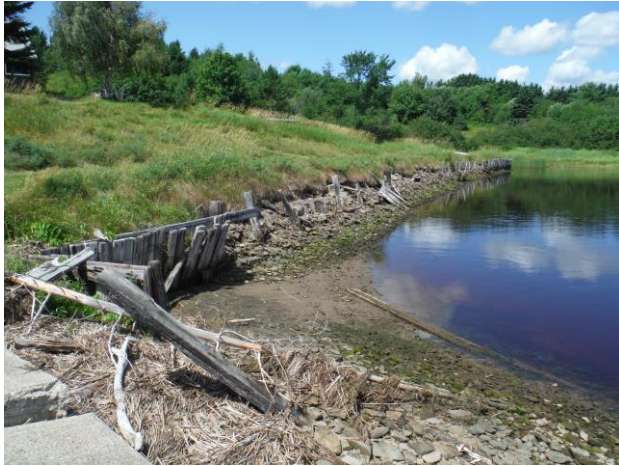
Pre-restoration photo displaying failing creosote wall (2012)
